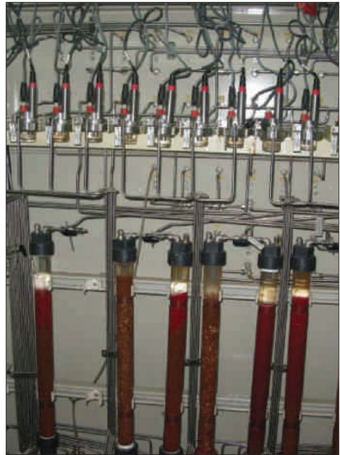
Figure 4: Rear view wet rack with sensors.
